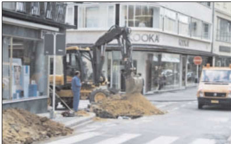
Picture 014 > Bad protected works In such situations, the risk of accidents is very high
